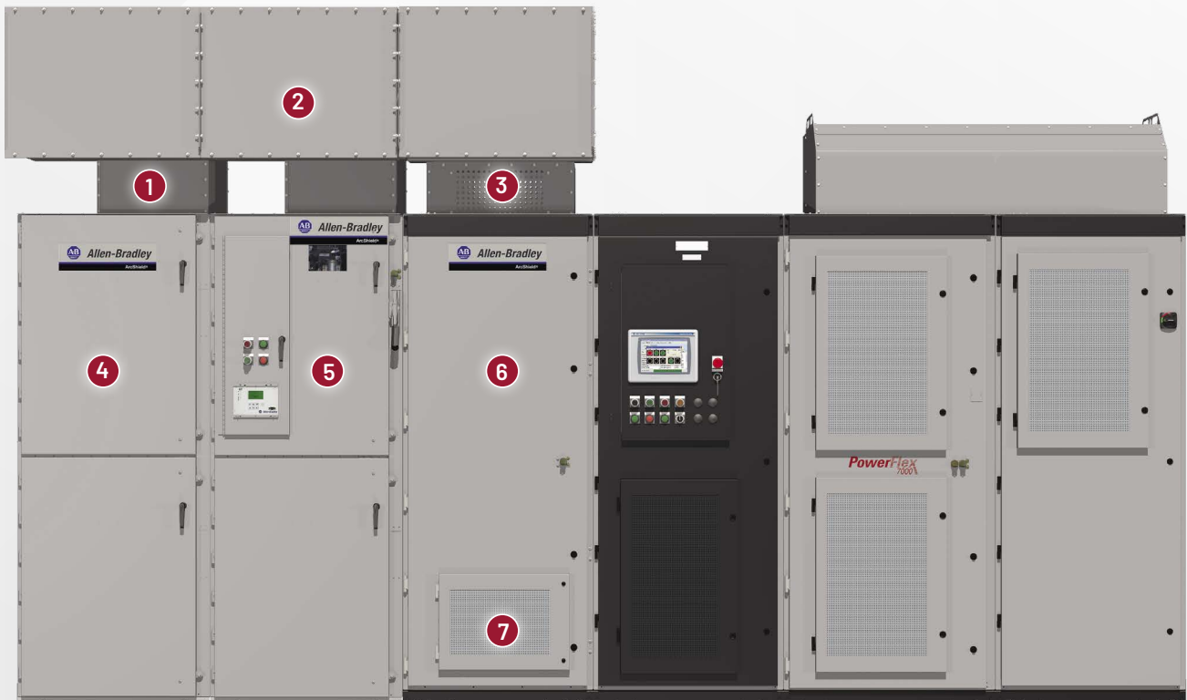
Fully integrated 50 kA rated PowerFlex 7000 Drive System with ArcShield Technology
